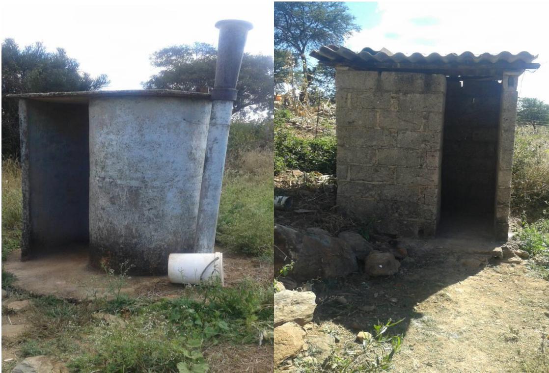
Figure 6. Examples of Dirty Toilets
