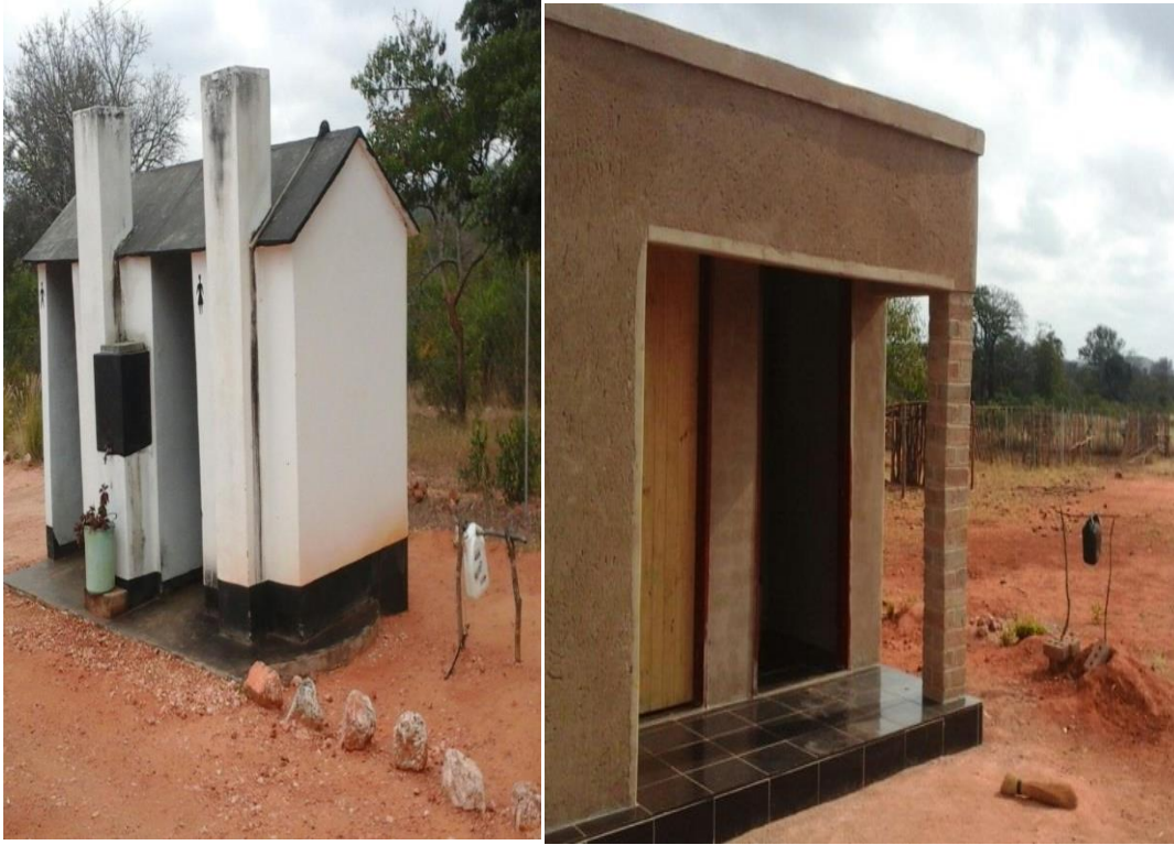
Figure 9. Examples of Designated Hand Washing Facilities
